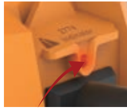
Warning light to show 277V input, preventing misuse of the connecting outlet
